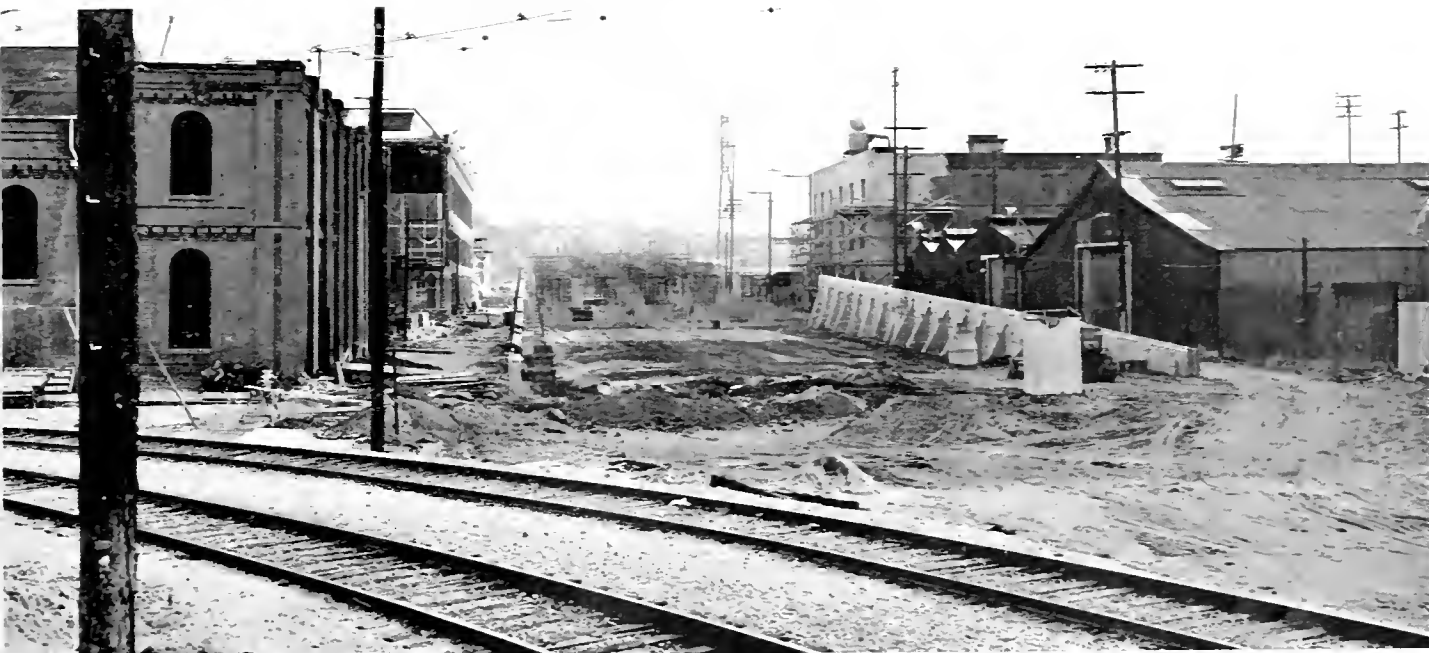
Construction begun on western approach to Aliso Street Bridge over Los Angeles River and distribution structure
